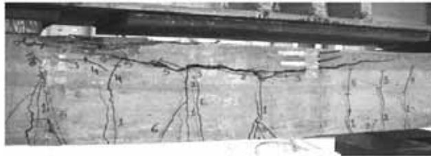
Fig. 5: Flexural Failure of Control Beam AH0
