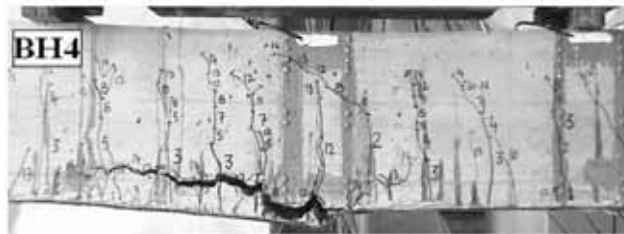
Fig. 6: Rupture of FRP in Beam BH4
