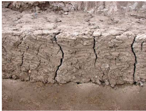
Fig. 4: Failure induced by water penetration down upward on Tous wall.
