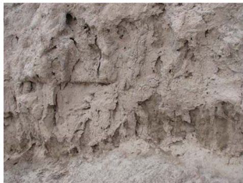
Fig. 7: Failure induced by wind accompanied by rain on Tous wall.
