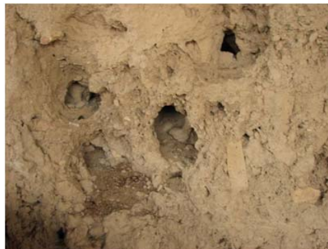
Fig. 6: Failure induced by rat activities on Tous wall.
