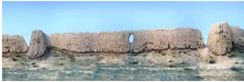
Fig. 5: Failure induced by water penetration up downward on Tous wall.
