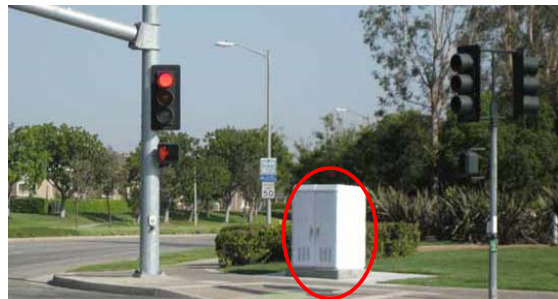
Fig. 3: PLC controller on a certain junction.
